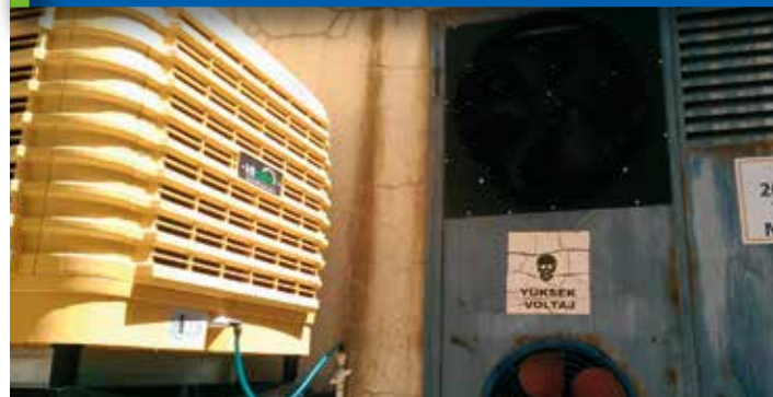
TRAFO ODASI / TRANSFORMER ROOM
