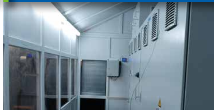
ELEKTRİK PANO ODASI / ELECTRIC CONTROL ROOM
