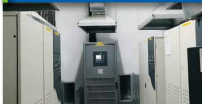
UPS ODASI / UPS ROOM
